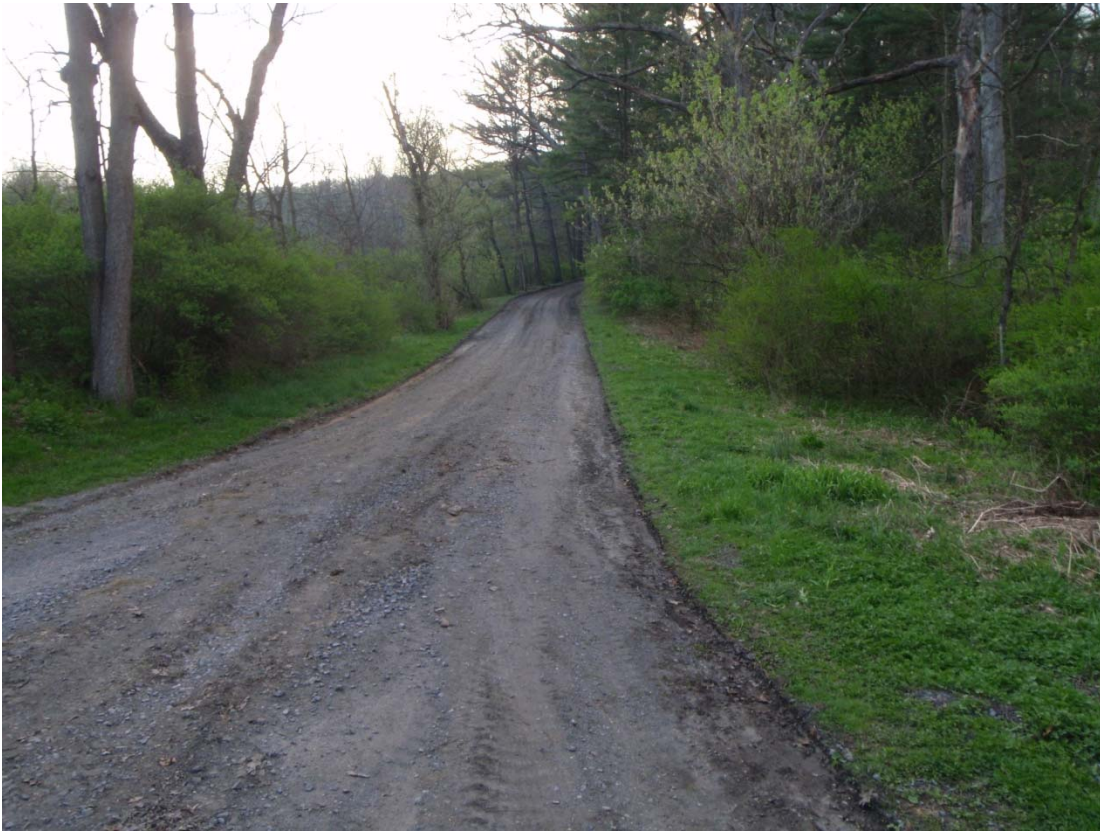
Figure 7. Photograph of Roadway Across Big Hollow with No Culvert (Gage 6 is located on the right side)
