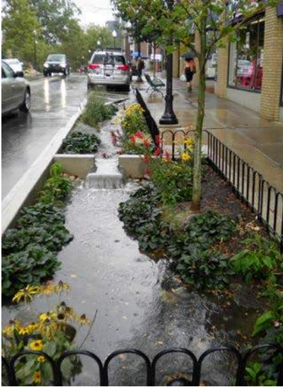
Photograph 2. One of two rain garden retrofit projects installed at the corner of Allen Street and Beaver Ave in the Borough of State College
