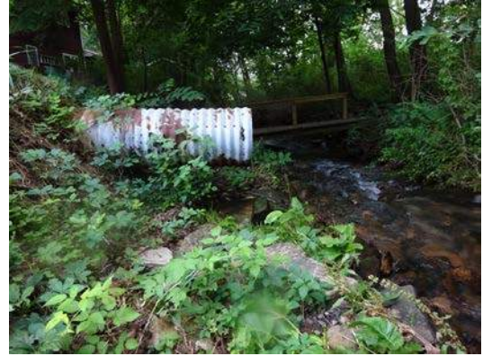
Photograph 3. Eroded streambank upstream end of reach
