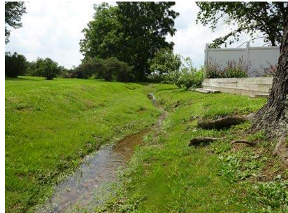
Photograph 2. Sediment deposition in channel
