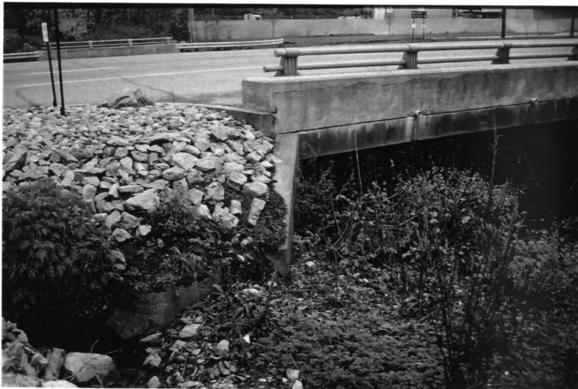
Photo 4A. Examples of stormwater input into Millbrook Marsh - Road runoff from E. College Ave. and Puddintown Road at the Thompson Run bridge, east side.
