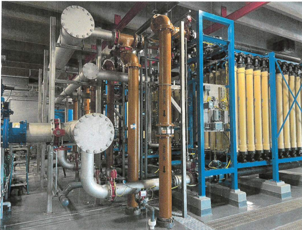
Membrane Filtration Mechanical Piping
