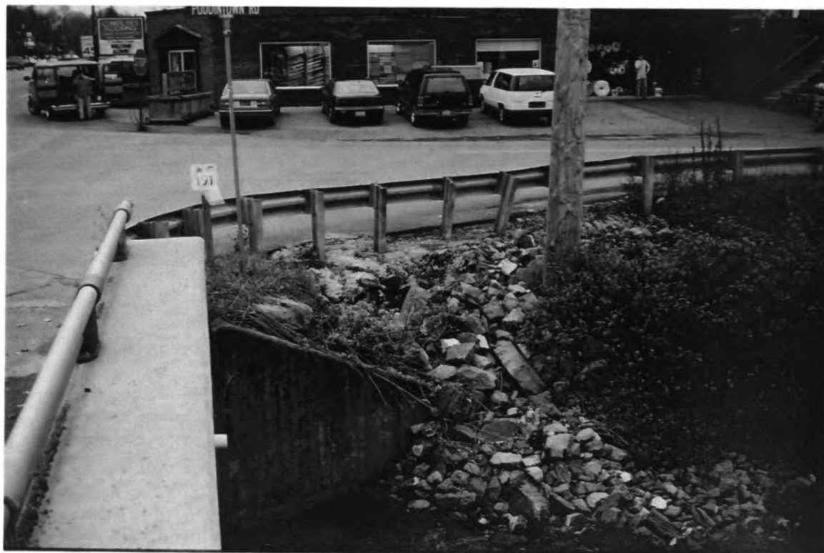
Photo 4B. Examples of stormwater input into Millbrook Marsh - Road runoff from E. College Ave. and Puddintown Road at the Thompson Run bridge, west side.
