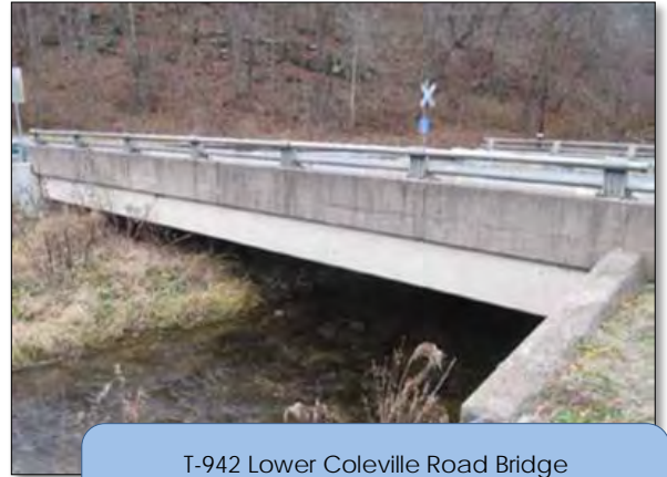
T-942 Lower Coleville Road Bridge Spring Township Centre County Bridge Bundle Application
